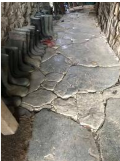
Cobbled passageway from garden gate to the back door of the Cottage
