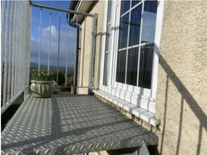
Platform and front door threshold
